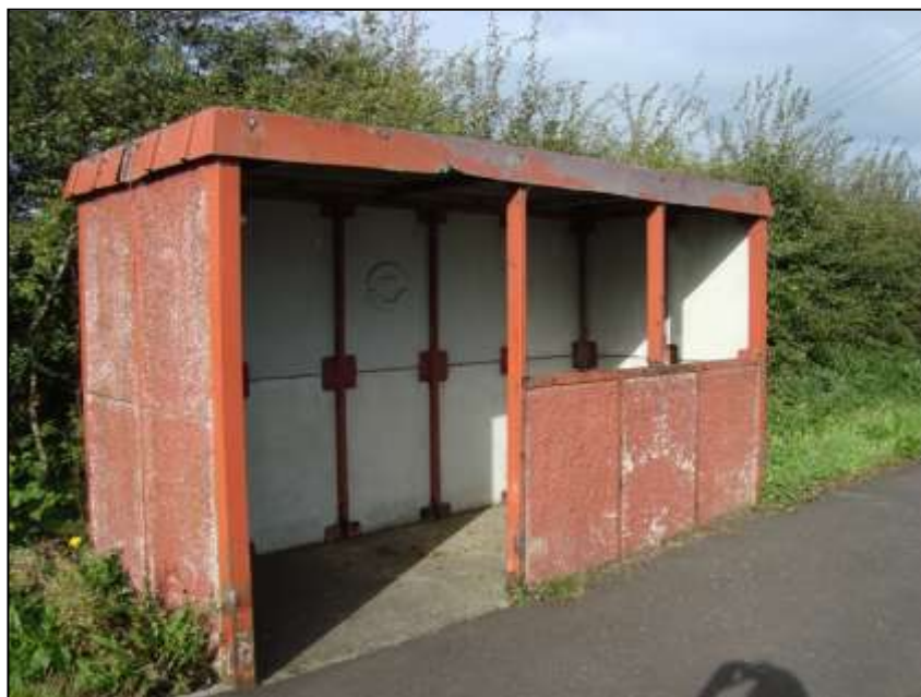
Plate 10: RCP Shelter at Garryduff Cross in a poor condition with rusting/decaying metal frame and holes in the roof.
