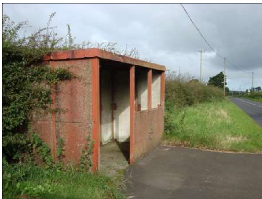
Plate 16: RCP Shelter at Heatherton Cross is another which could be considered for replacement with a Perspex shelter due to its deteriorating condition with holes in the roof, the floor breaking up and general disrepair.
